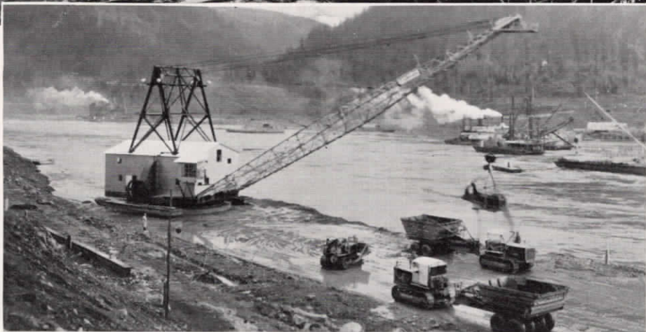
Foundation forms for the powerhouse at Bonneville Dam are shown in the top picture. A Monighan drag, with one of largest booms ever used, at work on river bed in the lower photograph.
