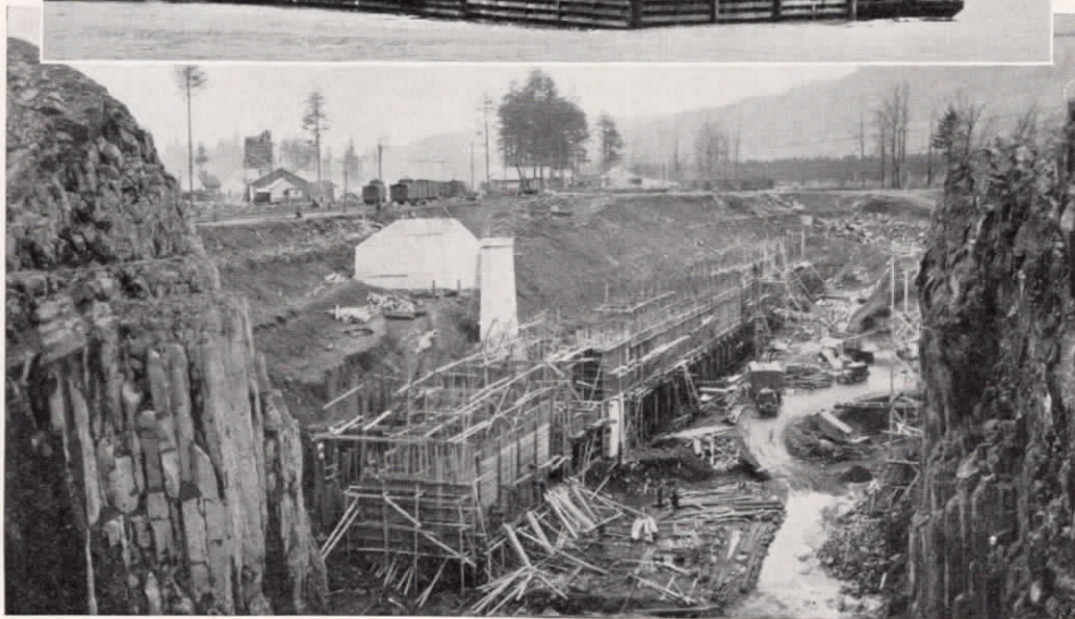
The first shore cribs on the Bonneville Dam work are shown under construction in the picture at the top; mid-river cribs are shown in center; and below, preliminary forms for the largest lift locks in the world—a rise of 59 feet will be accomplished.
