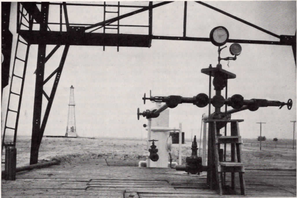
The above photograph, taken from the floor of Kernco No. 1, the Union Oil Company well that extended the Mountain View field nearly three miles, shows Kernco No. 2, 1000 feet distant, recently completed at a depth of 5546 feet with an initial flow of 3,240 barrels a day of 30.8 gravity clean oil.
