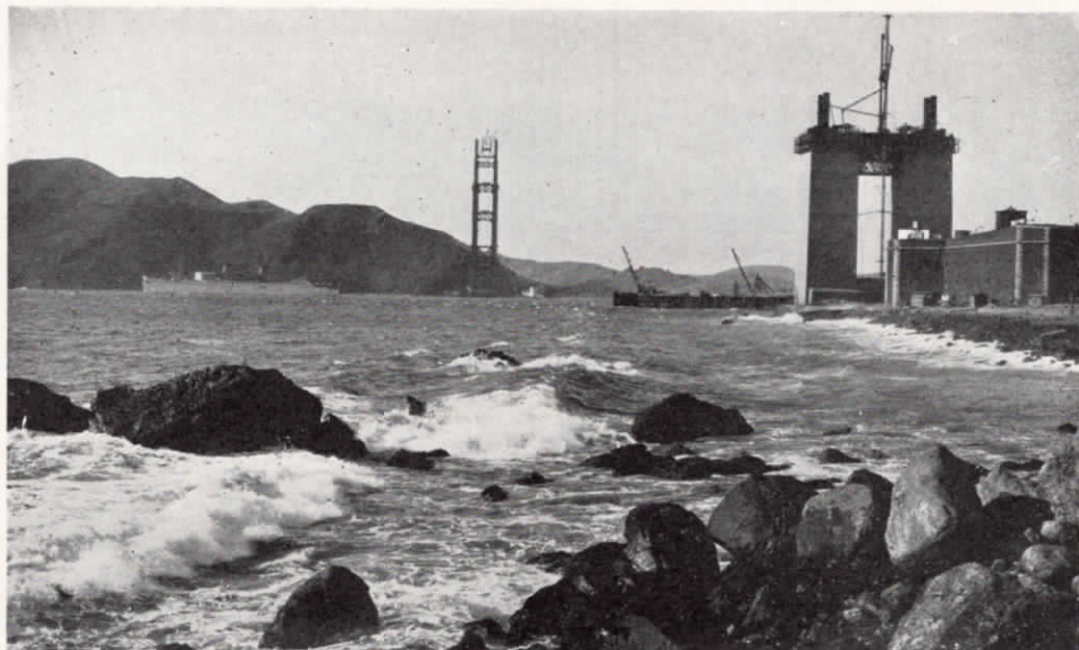
Where the Golden Gate is to be spanned. This view shows the Marin pier completed to its column height of 746 feet in the distance, while in the foreground is Fort Point, Pylon S-1 (now 170 feet high and scheduled to rise 250 feet) which is part of the San Francisco Pier anchorage, and in the middle distance is the wharf extending to the point where the fender of the San Francisco Pier is being constructed. This pier will rise to the same height as the one on the Marin County side, and will be the first ever built in the open sea.
