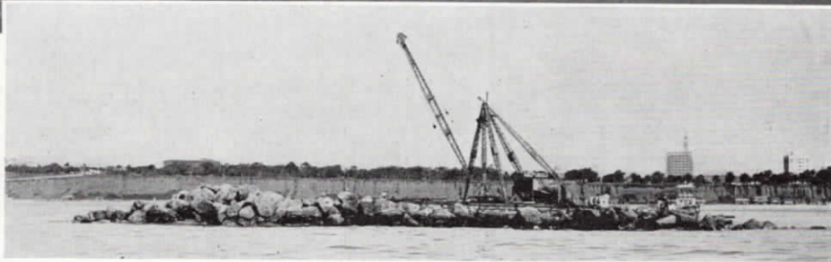
Santa Monica breakwater under construction and as it will appear when completed. The artist's picturization of the breakwater is drawn on a Spence aerial photograph of the bay. Extension of the pier is shown at the top and construction of the sea wall, below.
