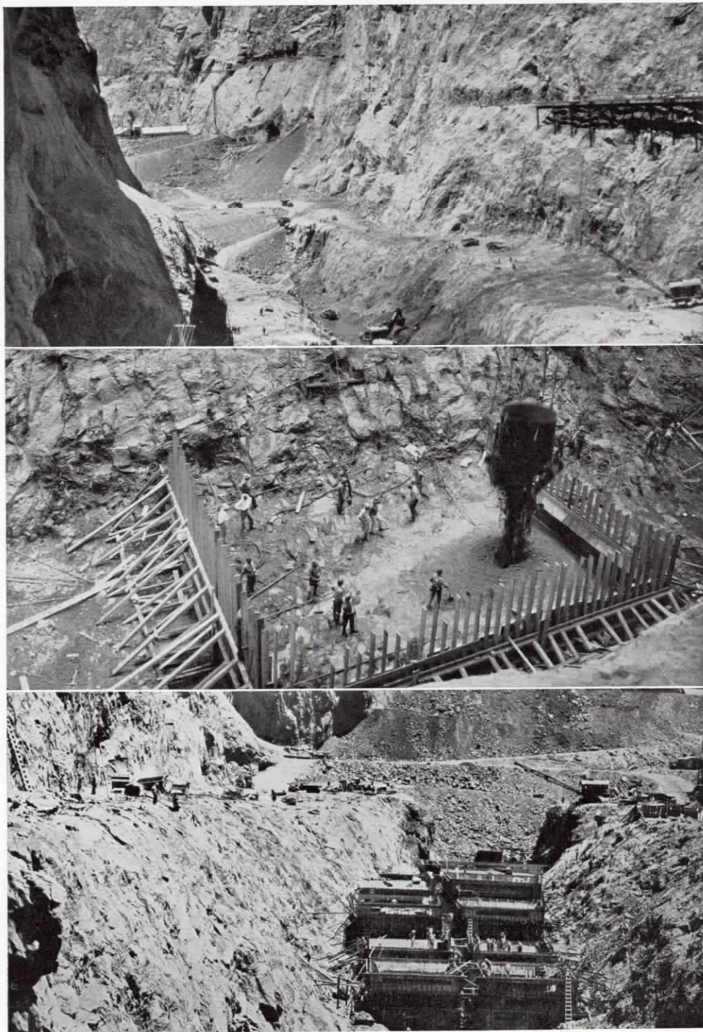
Progress photographs showing, at the top, the river bed excavated to bedrock for the dam foundation; center, first bucket of concrete being dumped, June 6, 1933, and bottom, first concrete forms as they appeared in the excavation below the old river level.
