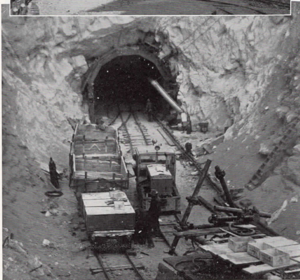
A new heavy duty capacity mucker, operated by Hunkin-Conkey Construction Co., on Hayfield Tunnel No. 1, is shown in the top picture. Below, tunneling equipment used on the job. Extreme left you see muck cars, gasoline powered dinky engine, and in right foreground, a jumbo upon which 12 drills are mounted for work at driving face of tunnels.
