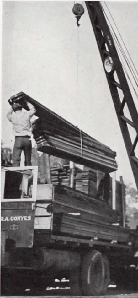
Trucking equipment of R. A. Conyes, hauling contractor for builders of Metropolitan Water District aqueduct.
