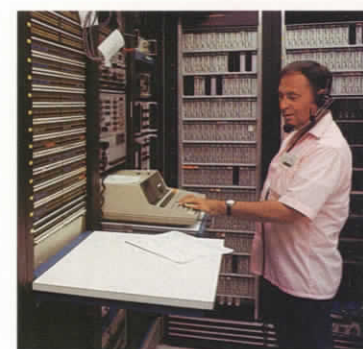
In the Telecommunications room at Unocal Center, computer-routed calls are transmitted over high-speed telephone lines, which send data as well as voice communications.
