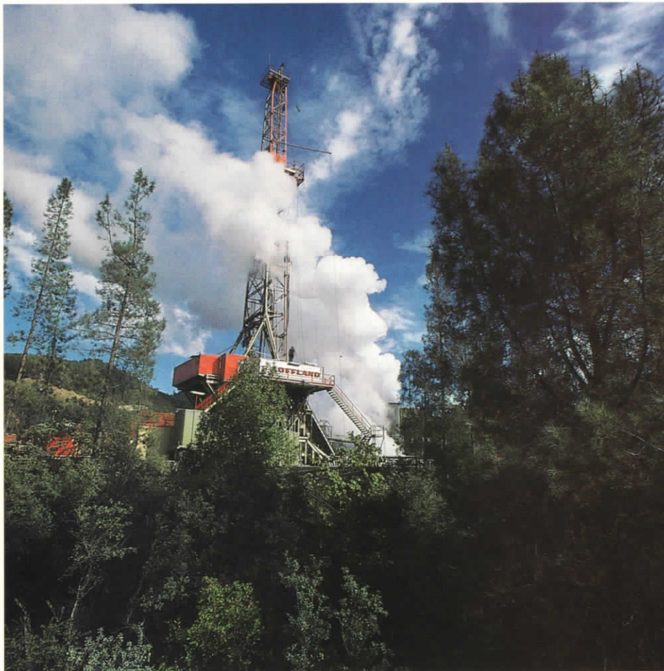
Opposite page, from left: Mike Riehle, Mike Dougherty, Terry Larson with secretary Roberta Treviranus. This page: Development drilling underway at Unocal's geothermal project at The Geysers, in Northern California. Alternative energy is one of the issue areas focused on by Unocal lobbyists.
