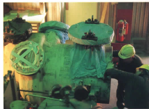
Designing, fabricating and installing the new urea process vessels was no small task. But the state-of-the-art equipment should last 20 to 30 years.
