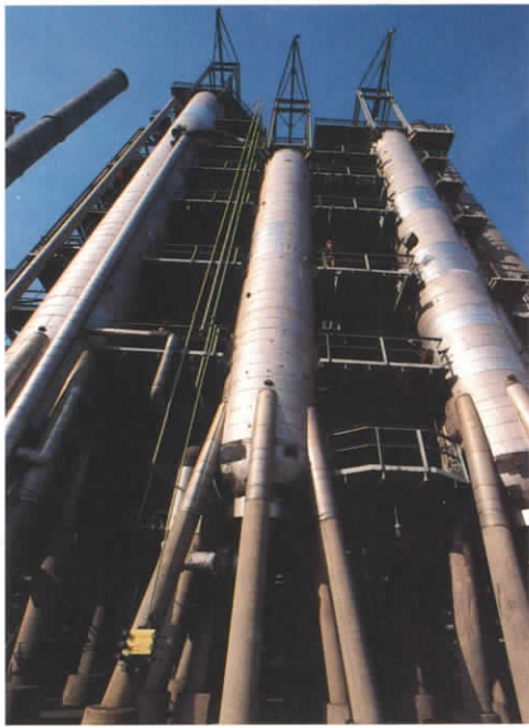
Unocal is a world leader in the development of petroleum refining technologies—among them, the company's patented Unicracking process. Pictured here is the Unicracker at Unocal's Los Angeles Refinery.
