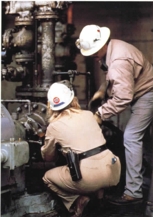
Outside, Rhonda Parkins and Dan Prieto (7) check the operation of one of the FCC's heater circulation pumps. Another pump functions quietly on its own (3).
