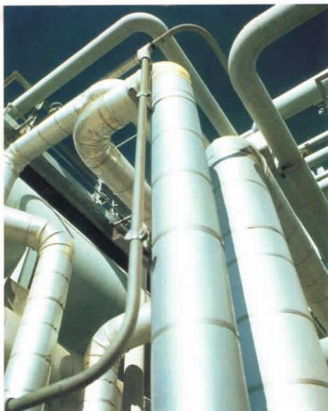
Above, a maze of pipes cuts through the sky at the Los Angeles refinery. Below right, the San Francisco plant's coker. "We're continually striving to improve and enhance product quality."
