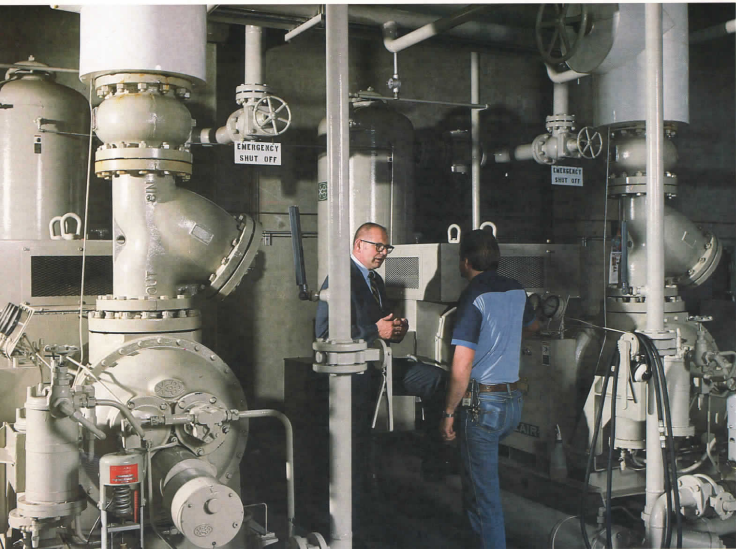
Hugh Haven (left) and Mike Brewer would not be standing between the ice-bank compressors without ear protection if the machines were operating. The noisy machines are housed in a concrete building, insulating them from both the research center's employees and neighbors. The compressors run during late night and early morning hours when the cost of energy is lowest.
