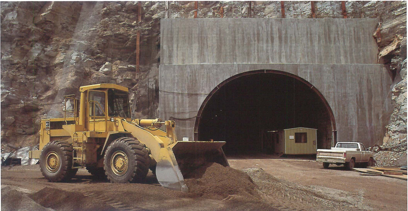
Mine entrance opening onto five-acre bench site where shale oil retorting facilities are being constructed.
